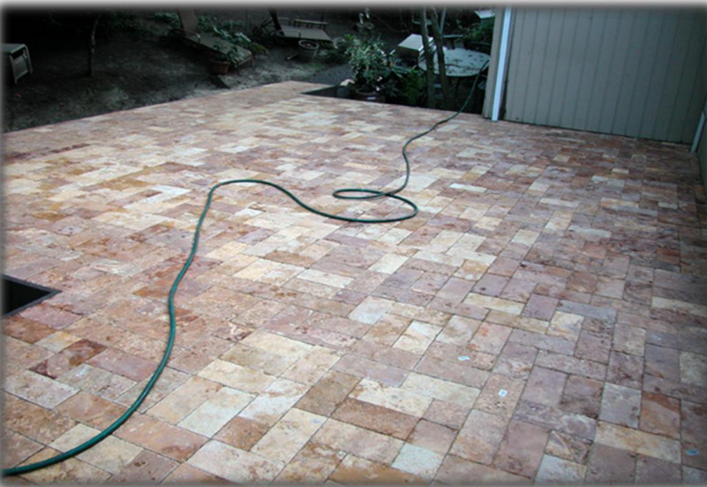
Figure 6 After installing the slate, John brushed polymeric sand over his deck. The above is a picture of the deck before he misted the sand.
